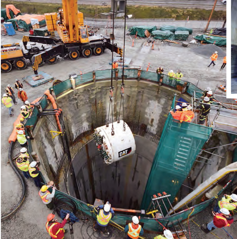
Above & below right: Work crews and the tunnel boring machine cutterhead entering the south shaft.
